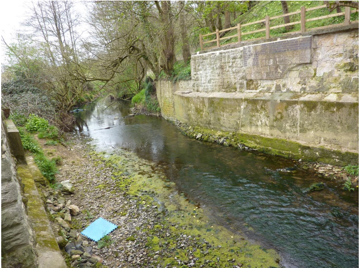
Figure 16: The shallow, exposed river channel through the old railway bridge footings would benefit from bankside cover (such as goat willows) on the RB
