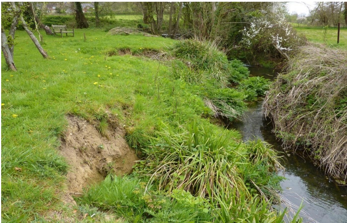
Figure 12: Two areas of bank failure on the main channel of the River Pitt in the Cole Manor Mill gardens, possibly associated with seepage from the higher-level leat
