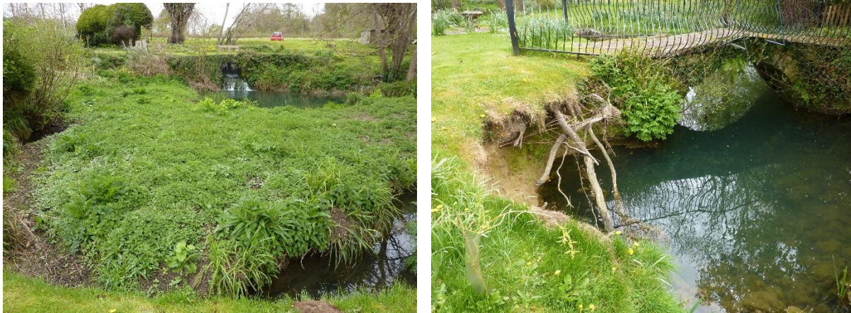
Figure 13: Cole Manor gardens: the silted ornamental pond (left - with a sluice gate from the mill leat visible in the background) and erosion caused by a back eddy from the abutments of a footbridge (right)
